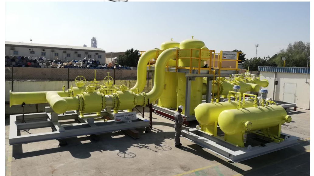
Assembled 2x100% Coalescing Separators & Drain Tanks
